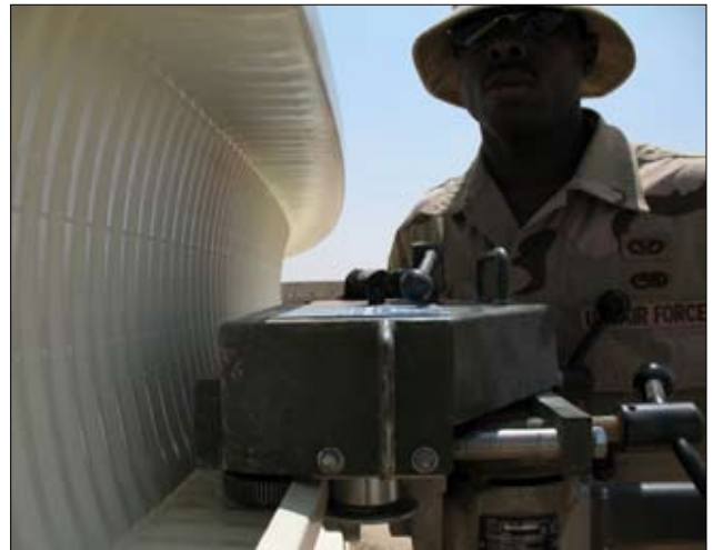
Photo by 165th Air Control Wing Public Affairs Office Staff Sgt. Randy Ellis a member of the 165th Civil Engineering Squadron deployed for 17 day to Nevatim Air Force Base in Israel, carefully uses a binding machine in the construction of the aircraft hangar. The squadron constructed meta aircraft shades for visiting American fighters.
